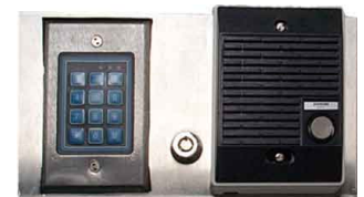
Install a key-switch & blank plate
